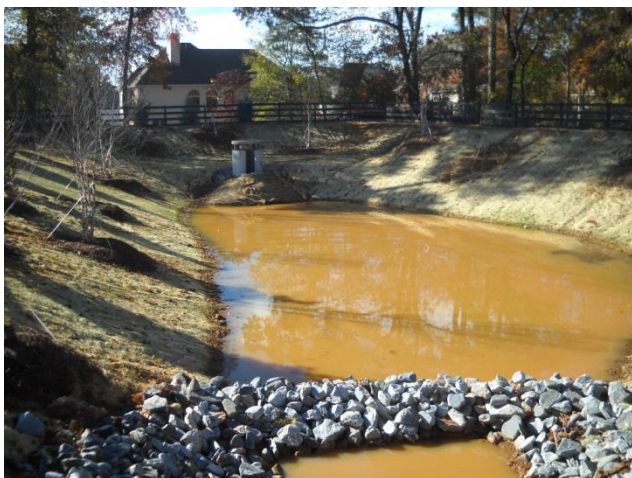
Standing water in dry pond
