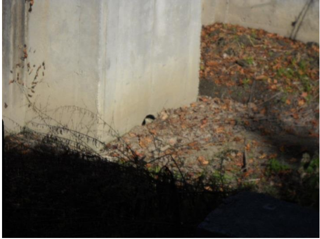
Accumulated silt clogging outlet pipe
