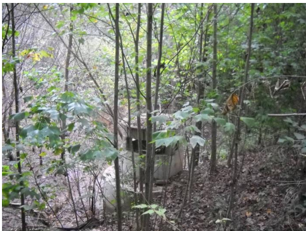
Undesirable tree growth on embankment slope
