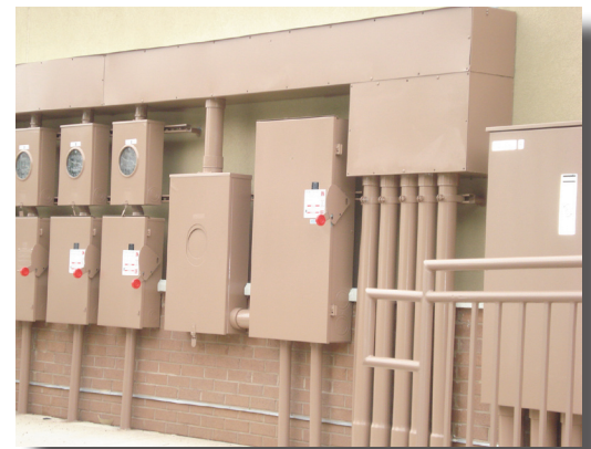
Utility meters should be painted to match the color of the building.
