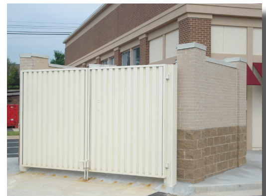
Dumpster walls shall be constructed of non-combustible brick or stone and is compatible with the design and color selections used on the principle building.
