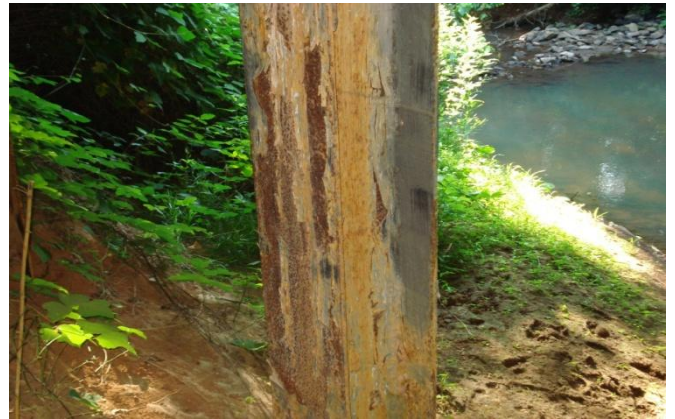
121-0698-0 – Epoxy Mastic peeling off
