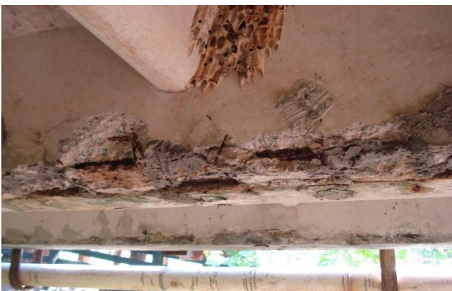
121-5009-0 – Main bars exposed due to spalling
