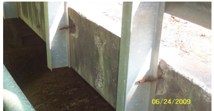
MLT04 – Guardrail anchor bolt spalling along Southside
