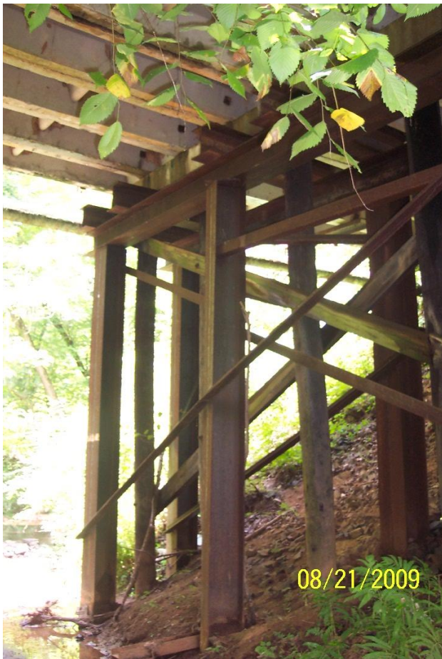
121-5015-0 – Twisted Steel H Pile
