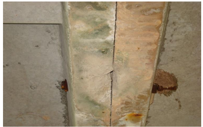
121-5013-0 – Spalling on edge of precast double tee
