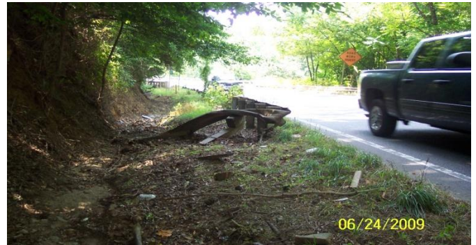
057-0029-0 – Guardrail damage Southwest Corner
