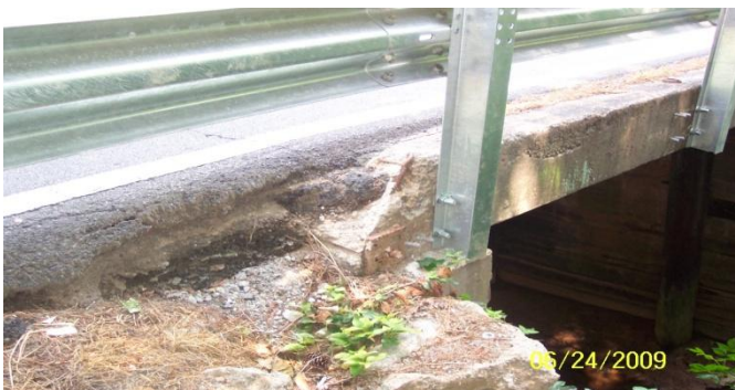
MLT01 – Concrete damage Southeast Corner
