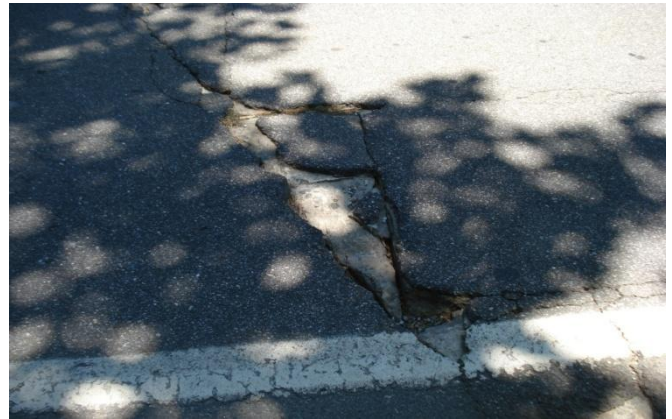
121-5003-0 – Crack between panel and asphalt
