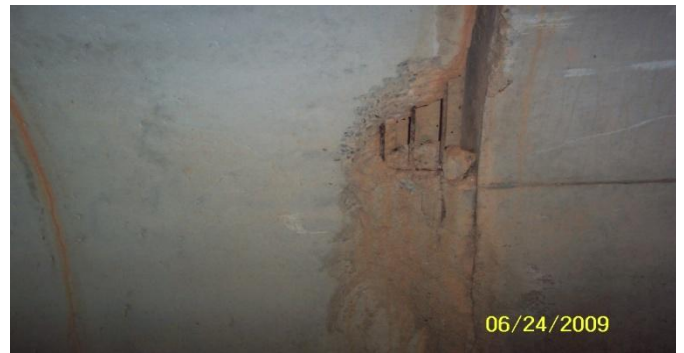
MLT06 – Spall location within pipe
