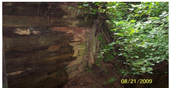
MLT01 – Timber Pile Damage Northwest Corner
