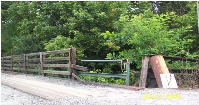
121-5002-0 – Damaged Fence South East Corner
