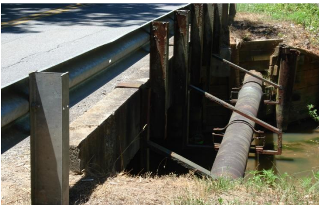
121-5003-0 – Post missing on NE corner
