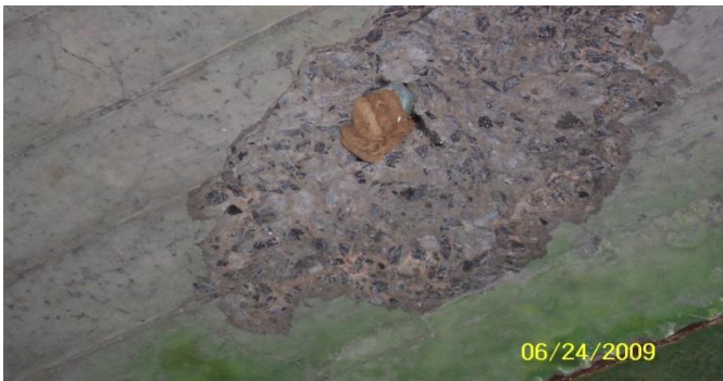
057-0029-0 – Spalling on deck from below
