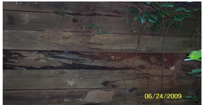
MLT01 – Timber wingwall damage Southeast Corner
