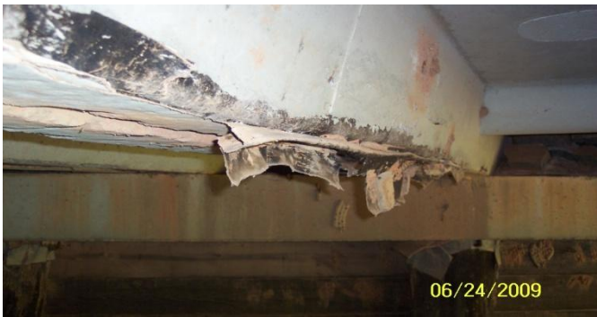
MLT04 – Fabric on underside of beam
