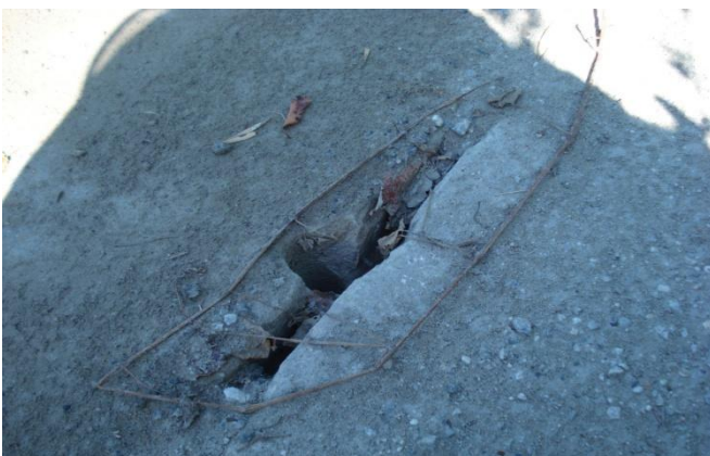
121-5013-0 – Drainage location with damage
