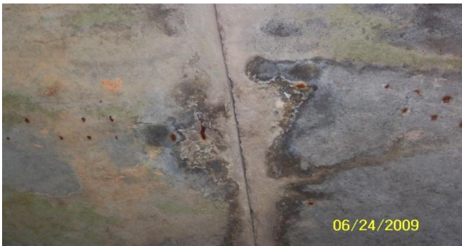
MLT01 – Spall location underside of beam
