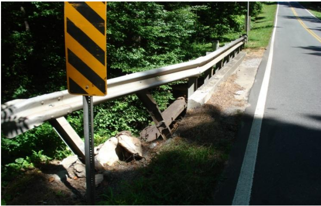
121-5202-0 – Damaged Guardrail on SW Corner
