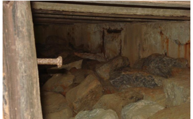
121-5014-0 Main rebar exposed due to spalling
