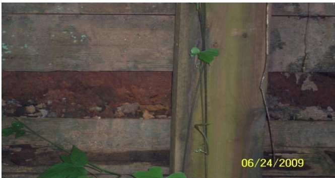
MLT05 – Timber wingwall damage Northeast Corner
