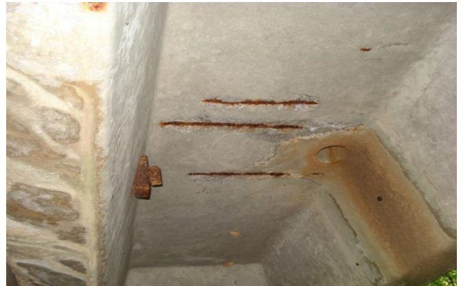
121-5004-0 – Minor spalling with previous patching
